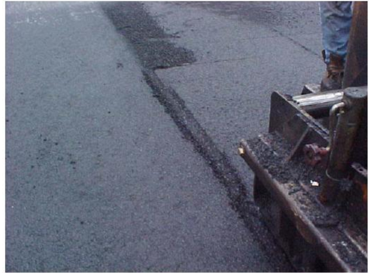
FIGURE 12 Excessive amount of overlap mix from Lane 2 over Lane 1, which creates the need for improper raking of the joint.
